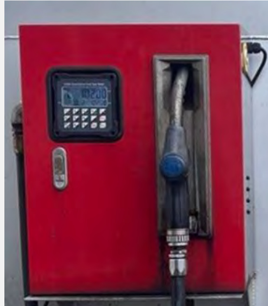
B20 storage tank with pump and meter
